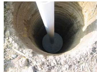
casing extended from lid to above surface
